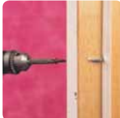
Drywall Screw Piercing Insulation
