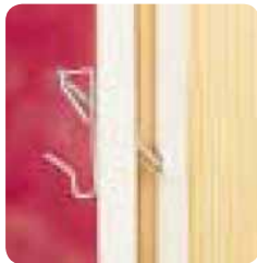
Nails or screws carelessly driven into walls
